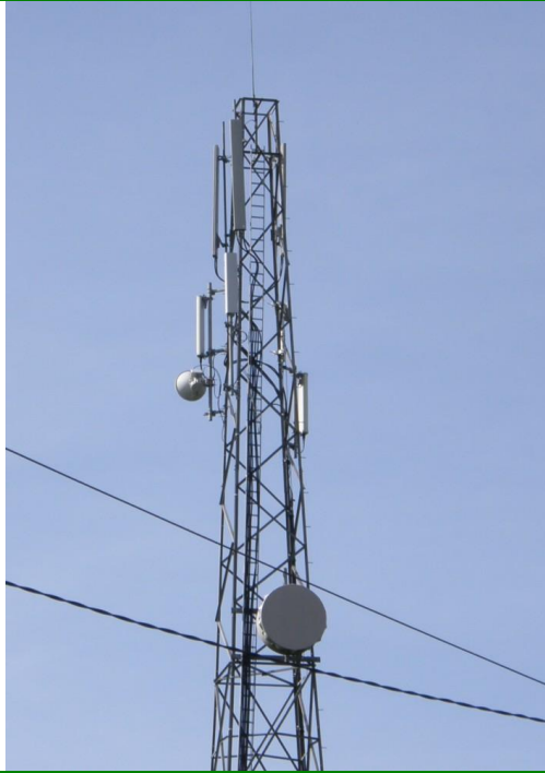
Transmitter Site Photo
